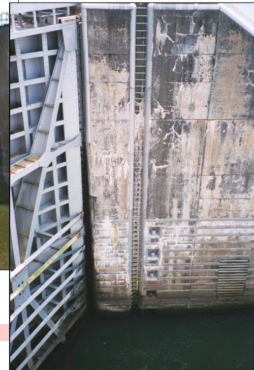
Concrete deterioration at Chickamauga
