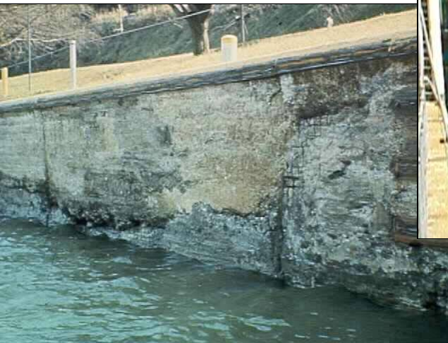
Crumbling lock wall, Lower Mon 3, opened in 1907
