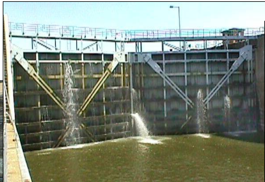
Leaking miter gates, Upper Miss Lock 19
