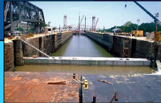
Dewatering and repairs of Inner Harbor Lock, New Orleans, which opened in 1923 for steamboats.
